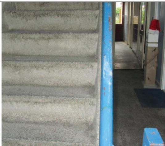
Foto 10. Detail schilderwerk trapleuning.
